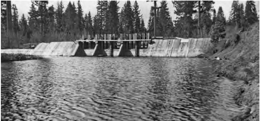
Figure 32 Timber buttress dam at the Lake Tahoe outlet built in 1870 [25] (University of Nevada Special Collections)
